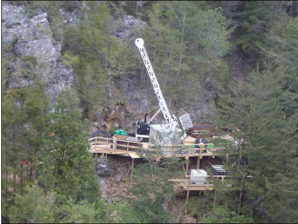
Figure 5-4: Alton Drilling drill rig setup in challenging conditions at Reefton. A similar setup could be used for Glamorgan drilling.
